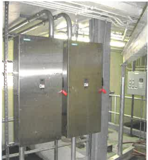
New 400 Amp Safety Switches
