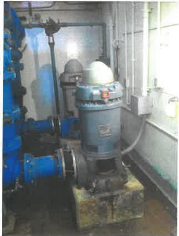
Old 75 HP VT Pumps
